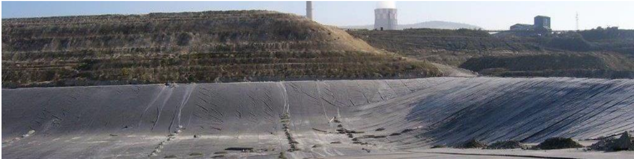
Figure 5 - Liner on bottom and on lateral side of initially embankment of ash disposal site
