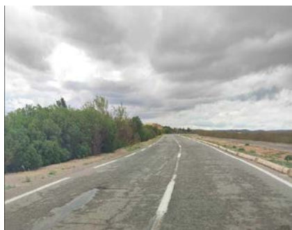
Figure 4 – Longitudinal and transverse medium cracking observed on the pavement surface
