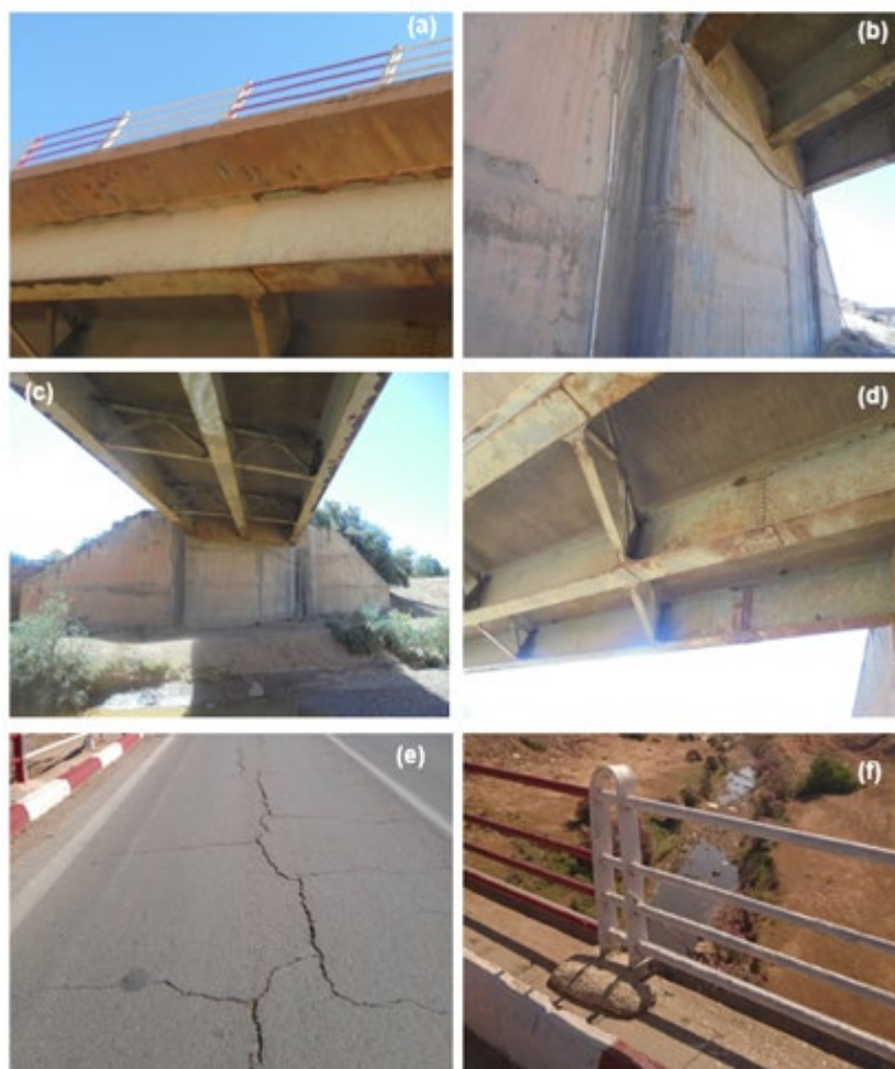
Figure 4 – Images depicting the extent of bridge damage: a) intrados of a cantilevered slab, b) abutment 02, c) main beams, d) cross frame, e) pavement, f) barrier
