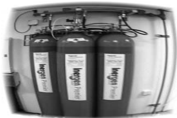
Figure 5. Inergen fire extinguisher (figure source: http://www.firesuppression.co.uk/inergen.aspx ).
