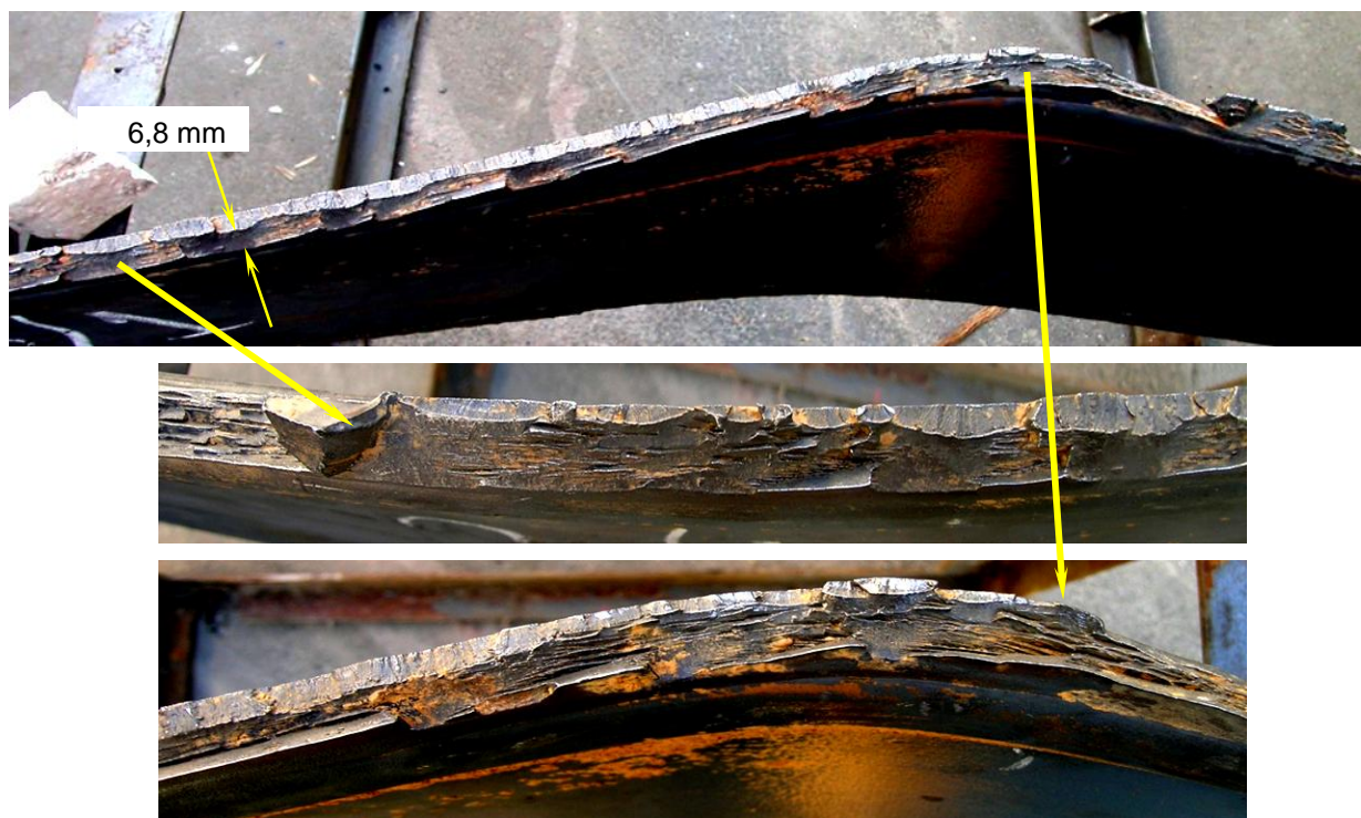
Figure 5. Sharp bend of pipe A (templet 3/1) ~470 mm long and ~6,8 mm maximum depth Slika 5. Oštra krivina cevi A (tempor 3/1) ~470 mm dužine i ~6,8 mm maksimalne dubine
