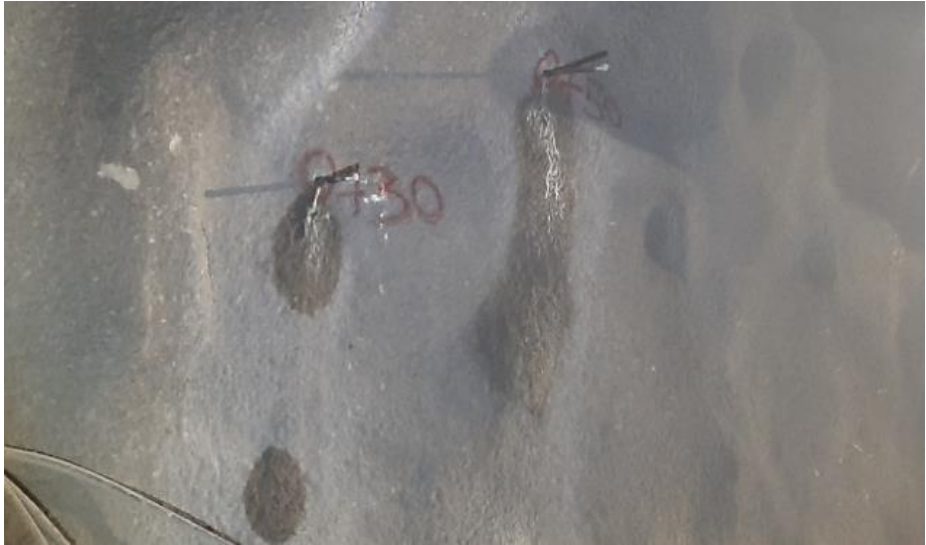
Figure 2. The presence of water in the form of wetting
