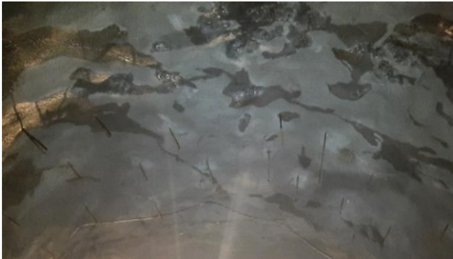
Figure 13. Display of installed short anchors for the purpose of diverting groundwater inflow
