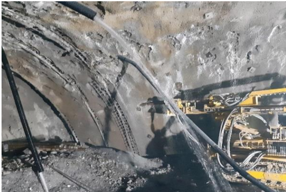
Figure 11. Water inflow through built-in drainage holes
