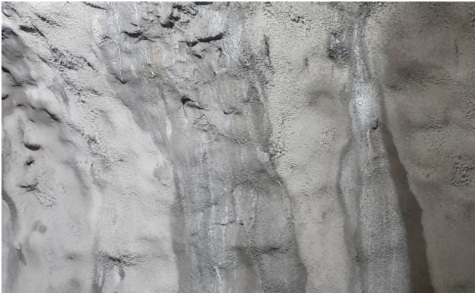
Figure 3. The presence of water in the form of wetting
