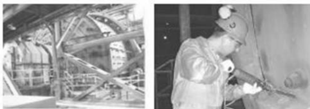
Figure 13. General view of one of the grinding mills that was treated by UP (left) and application of UP for rehabilitation of a weldment region in the grinding mill (right).
