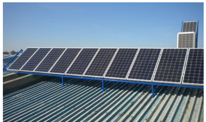
Figure 1. Solar modules inclined at 32° towards the South on the roof of the building in Niš.
