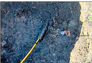
Figure 2. optical cable encased in 40mm PE protective tube
