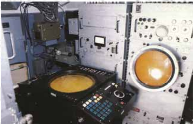
Figure 75. Control board of the surveillance-acquisition radar P-15 in the SONIC system
