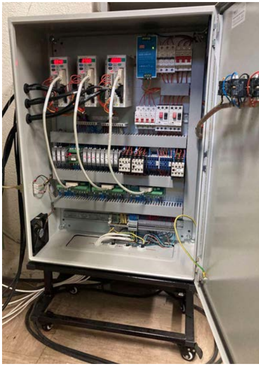
Figure 10. Control unit of the CNC machine - Profilator 100
