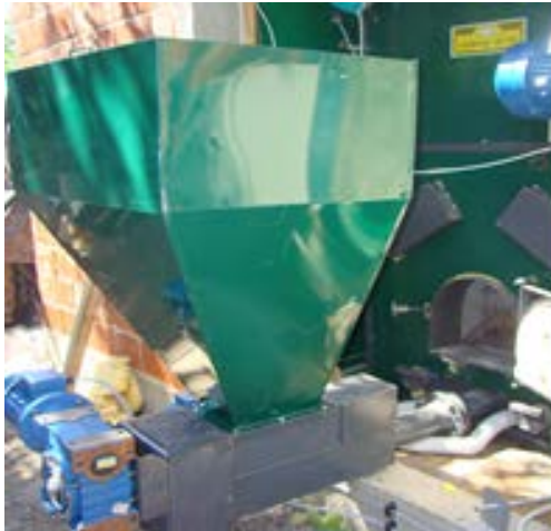
Fig. 1. Heat generator "XY", location A
