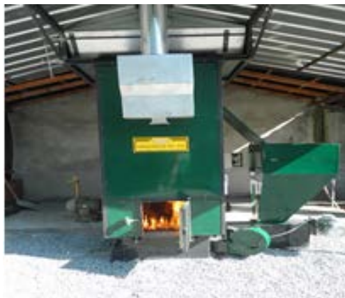
Fig. 2. Heat generator "YX", location B
