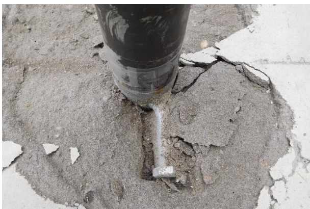
Figure 18. Concrete failure of stud connection
