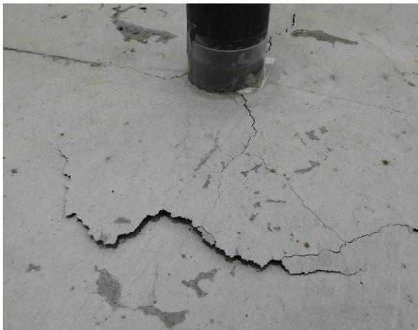
Figure 19. Early concrete surface cracking
