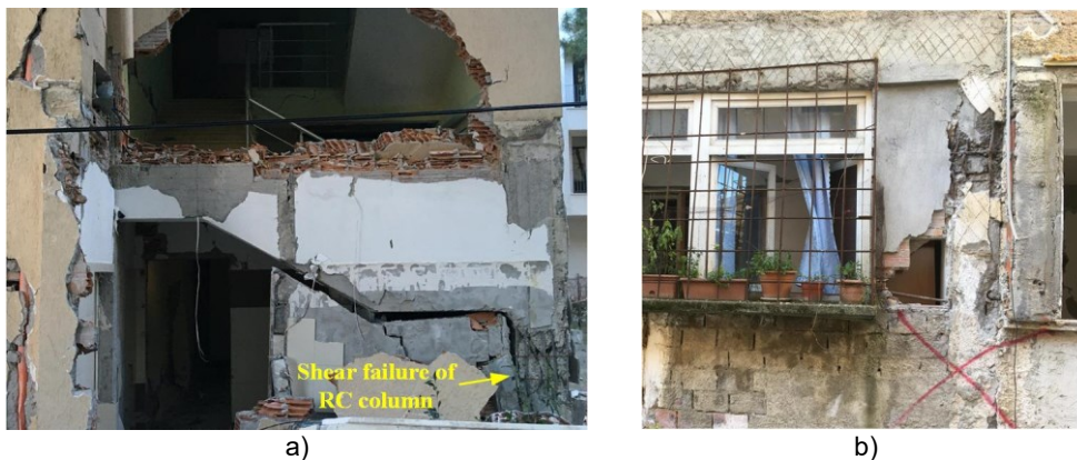
Figure 4. Examples of RC column damage due to “short column” effect in the Albania earthquake caused by: a) intermediate staircase landing, b) partial masonry infill due to openings
