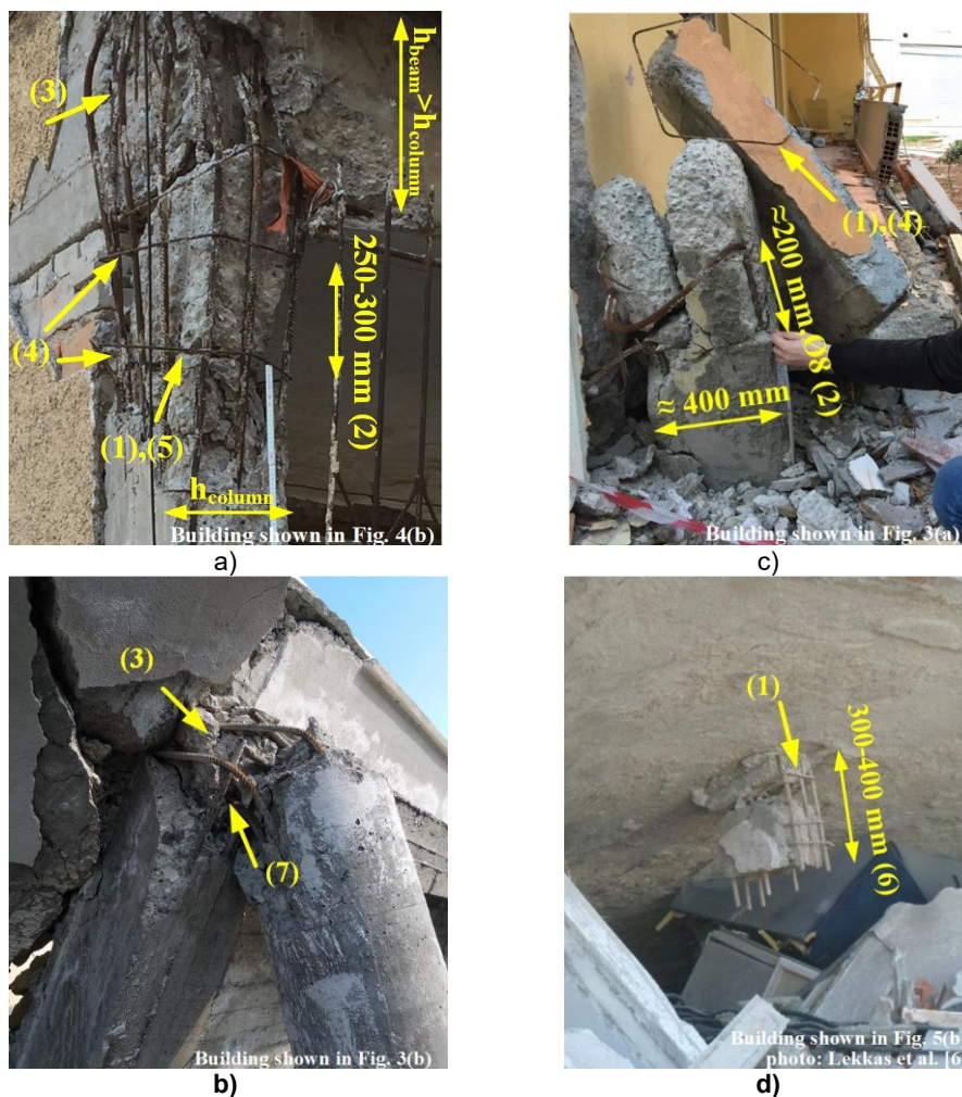
Figure 6. Examples of inadequate detailing of reinforcement in RC columns and beams
