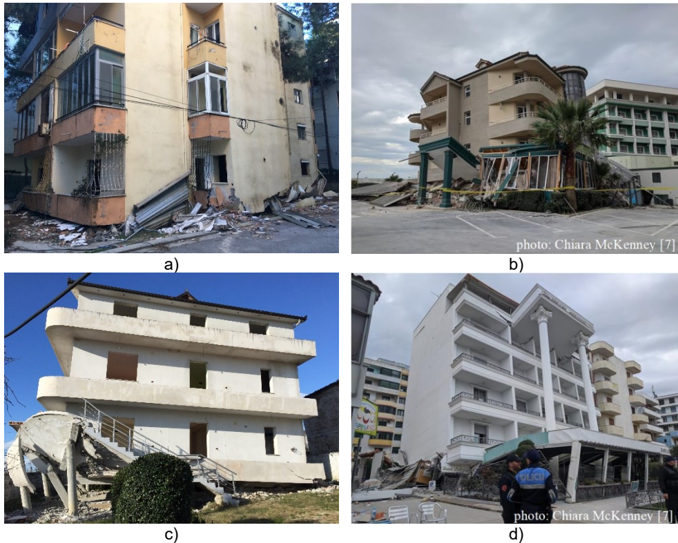
Figure 3. Examples of building collapses due to “soft storey” effect in the November 26, 2019
