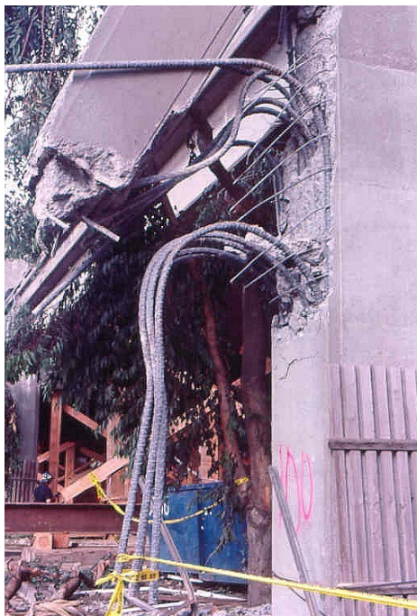
Figure 11 – a. Cypress Viaduct, Oakland
