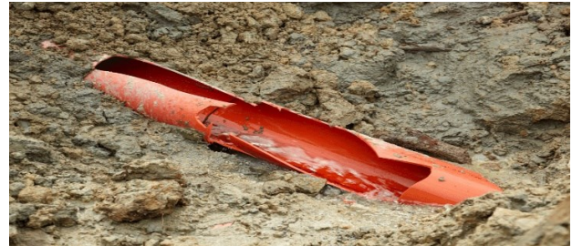
Figure 1. Failure due to deflection
