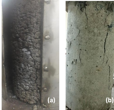
Figure 2. Cracks in column members(a) Diagonal Cracks (b) Splitting Cracks
