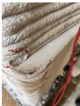
Figure 17. The local destruction of segments
