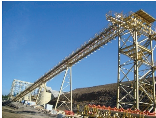
b) Belt conveyer with high-rise trestle
