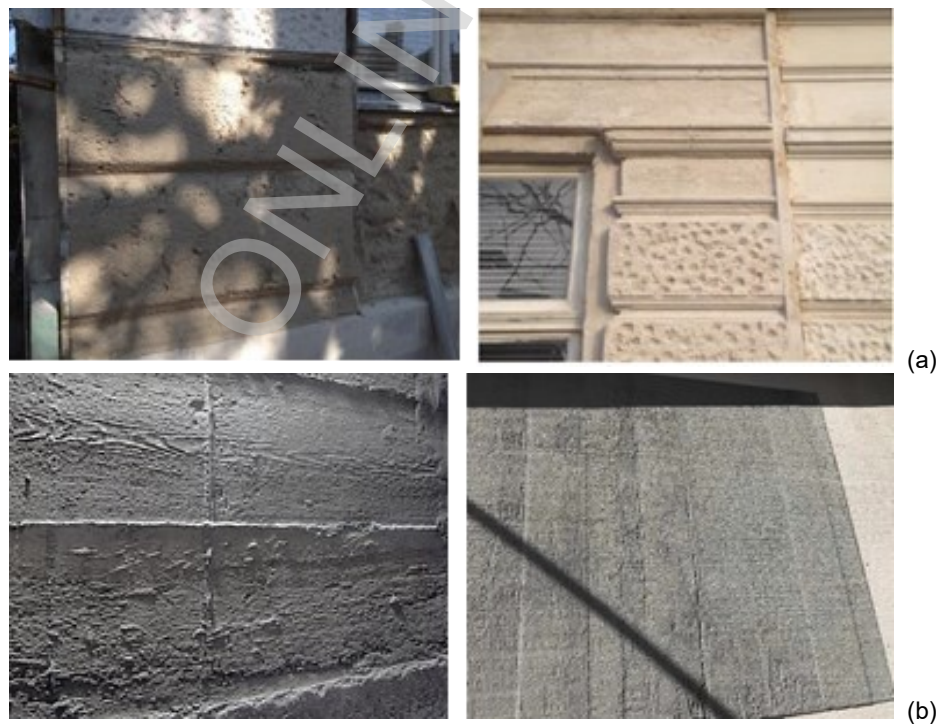
Figure 2. Visual comparison of façades in case of original materials and aerogel plaster application: (a) Renaissance building façade; (b) natural concrete façade
