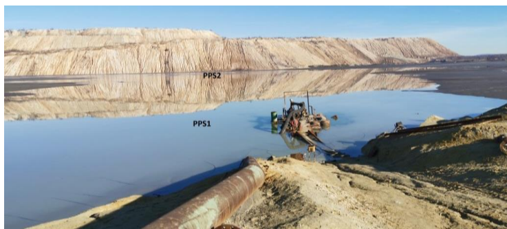
Figure 4 Existing and designed location of the floating pumping station, tailing dump RTH
