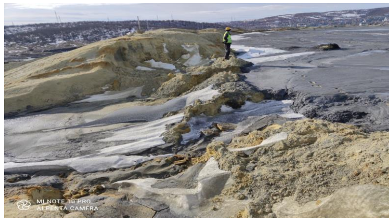
Figure 3 Completely eroded crown of the Dam 2 where the first serious overflows where the observed water and silt over the crown and downstream slope were recorded on January 29, 2021
