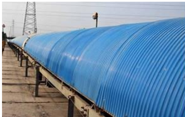
Figure 3 View of a belt conveyor
