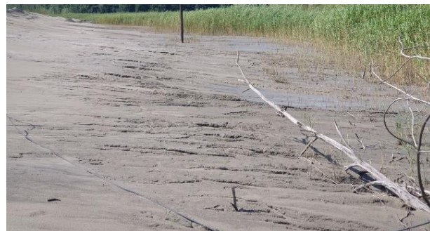
Figure 3 Effect of water erosion on the outer slope of the Dam 6, August 2023
