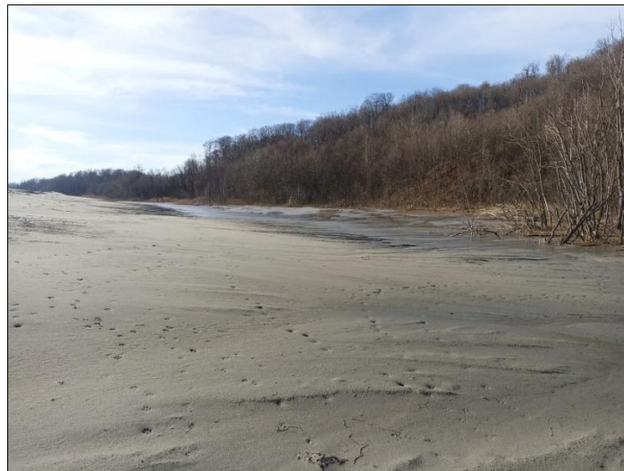
Figure 2 State of the external slope of the embankment
