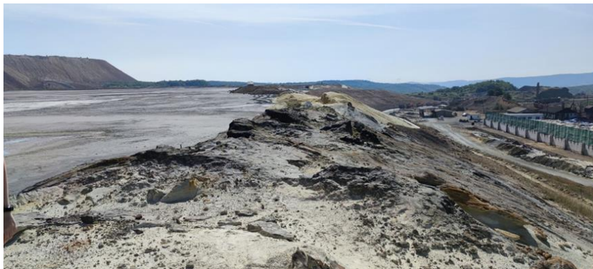
Figure 2 Detail of the endangered part of the embankment between PPS and dam 2, flotation tailing dump RTH, 2021
