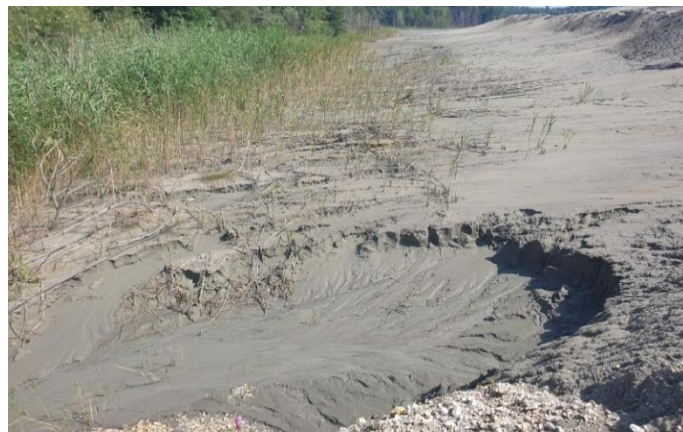
Figure 4 Effect of water erosion on the outer slope of the Dam 6, August 2023
