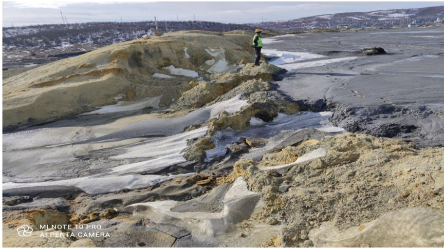
Figure 3 Completely eroded crown of the Dam 2 where the first serious overflows of water and sludge were observed over the crown and downstream slope, January 29, 2021
