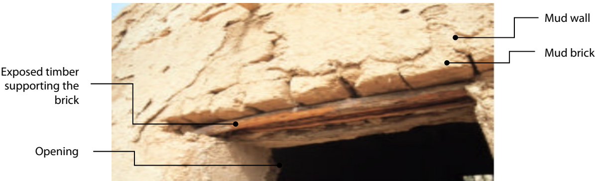
Figure 1: Lintel supported with an exposed timber
