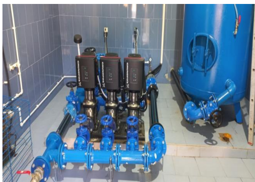
Slika 14. Pumpna stanica Kolut Figure 14. Pumping station Kolut
