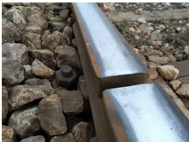
Fig. 2. Deformation of the rail's head (condition before reconstruction of superstructure)
