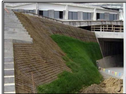
Figure 2 Reinforcement of supporting slopes with a geogrid, with the additional help of natural vegetation
