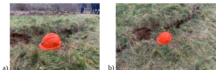
Figure 2. Cracks (a) and material settlement (b)
