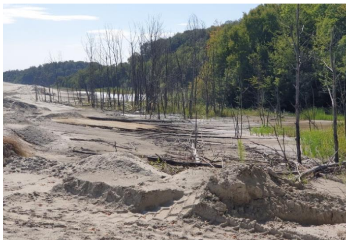
Figure 1. Discharge of material from the dam body in the seepage front zone on the outer slope of embankment in the Sector no. 6, Valja Fundata flotation tailing dump
