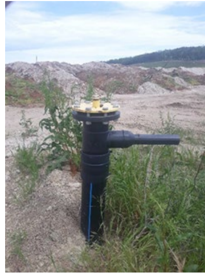
b) View of the horizontal connection of biogas degassing pipes
