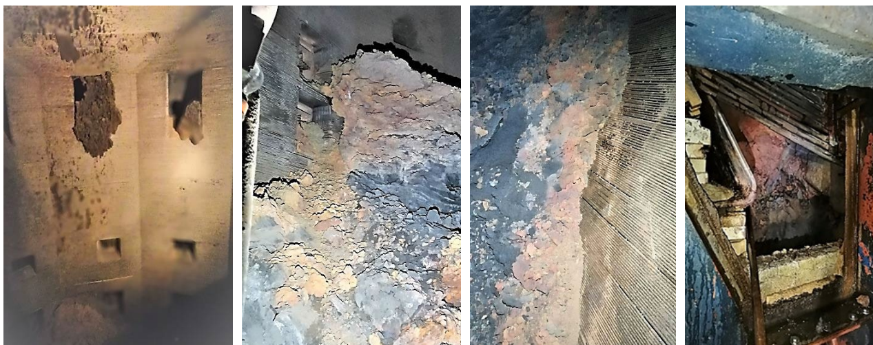
Figure 6. Slagging in the boiler furnace
