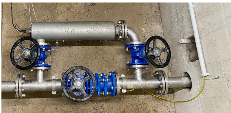
Slika 2. Primer tipične instalacije UV reaktora na vodovodnom sistemu Figure 2. View of typical UV disinfection system installation
