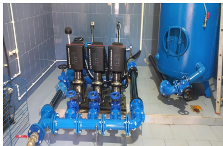
Slika 12. Pumpna stanica Kolut Figure 12. Pumping station Kolut
