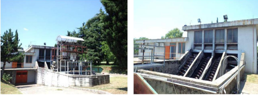
Slika 3. Ulaz u PPOV sa grubom rešetkom i pužnim pumpama Figure 3. Entrance to the WWTP with coarse grating and screw pumps
