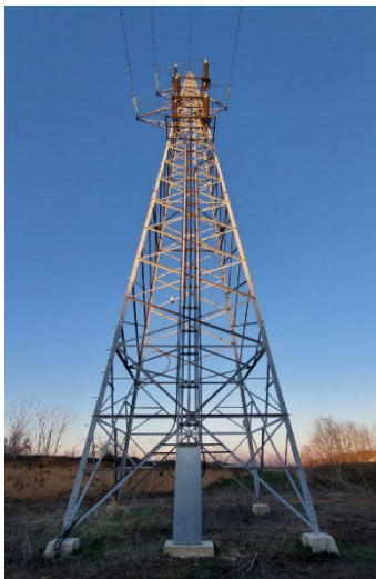
Figure 1. The tower at the transition point between the overhead and underground sections
