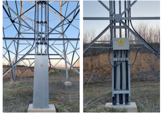
Figure 2. Cables descending into the ground, shown from the front side (a) and from the back (b)
