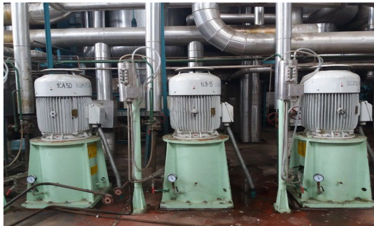
Fig. 1. I0 Condensate Pumps
