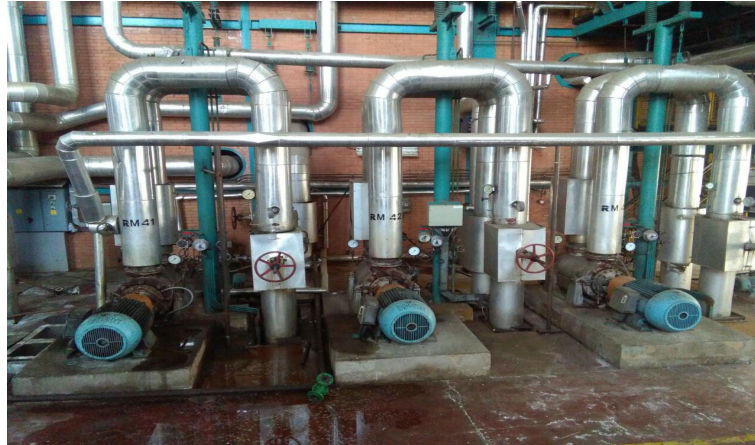
Fig. 2. IIO Condensate Pumps
