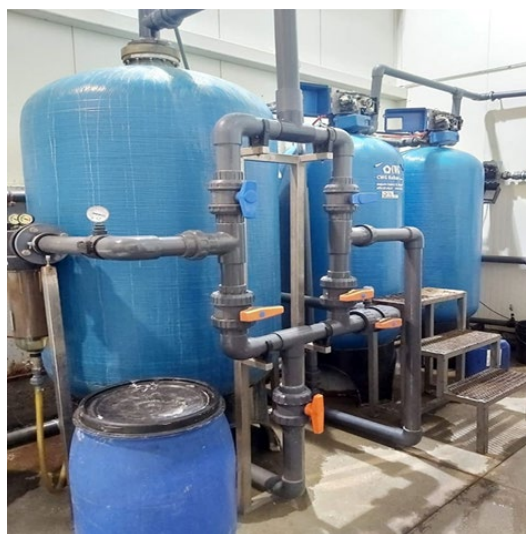
Fig. 2. Pre-sand filter, sand filter and scavengers
